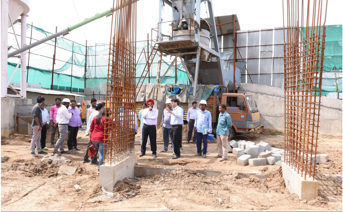
CEO, CGEWHO & Dy. Director (Tech), CGEWHO Inspecting Work Progress in 'D' Block
